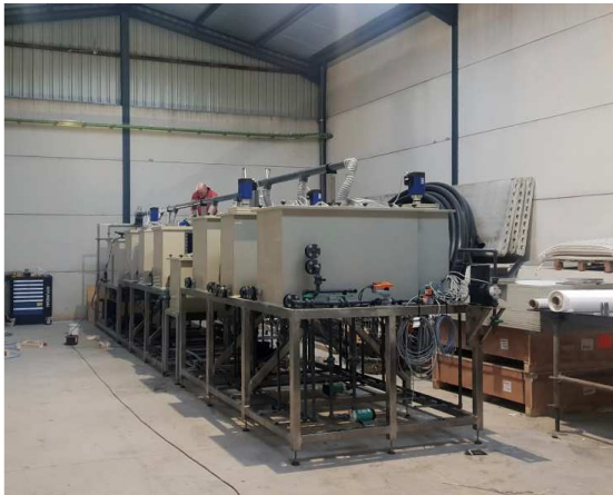
Copper SX circuit
